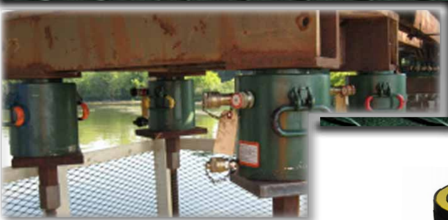
These 100 ton RCD cylinders are being used to construct grid sections for a bridge being built over the Susquehanna River at the mouth of the Chesapeake Bay.
